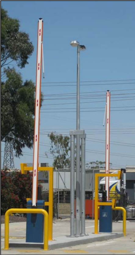
12x Boom Gates installed on one site w/ Traffic Light providing
